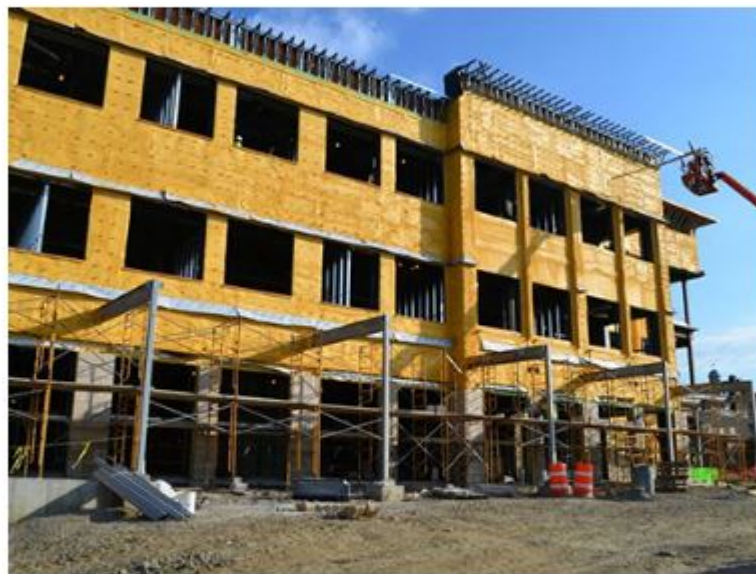
The $13 million build-to-suit corporate operations center for LCNB National Bank is located at 105 North Broadway, halfway between Cincinnati and Dayton.
